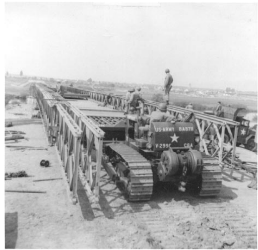
Construction of Bailey M-2 (triple/single) bridge during 37th Engineer Group panel bridge competition on Main River near Hanau, Germany, August 1960.
